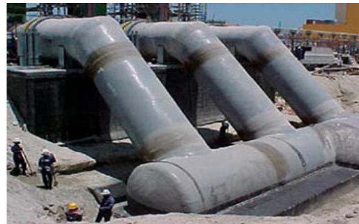
FRP Piping Manifold Desalination
